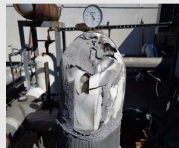
Deteriorated insulation on chilled water piping will all be replaced
