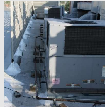
Aging HVAC equipment at Fire Station 55
