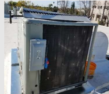
Aging HVAC units are in need of replacement
