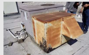
Package rooftop HVAC units are past useful life and need replacement
