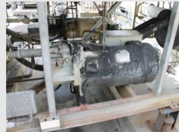
Signs of age on the existing chiller
