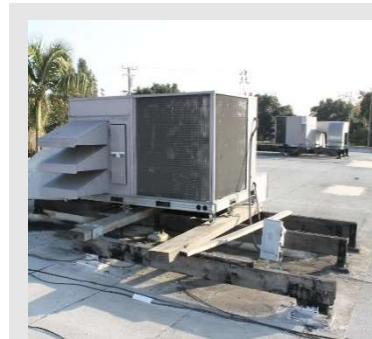
HVAC units at Hollifield Community Center are in poor condition with support framing in extremely poor condition
