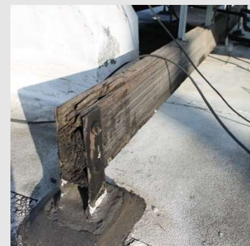
Example of the rotten wood framing supporting HVAC units above the Hollifield Community Center library
