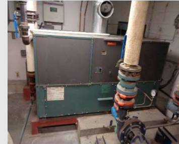
Existing Raypak boiler is nearing end of life and is ready for planned replacement
