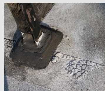
Further bubbling and cracking
