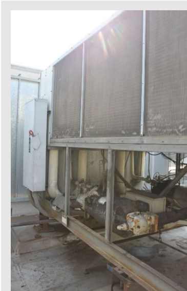
Side view of the existing chiller at Montebello Police Department
