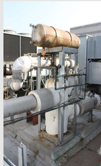
The existing pump skid, including pumps, air
