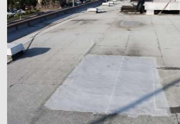
Significant patchwork at Holifield Community Center
