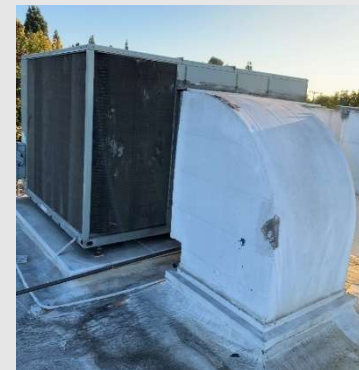
Aging unit serving City Council chambers
