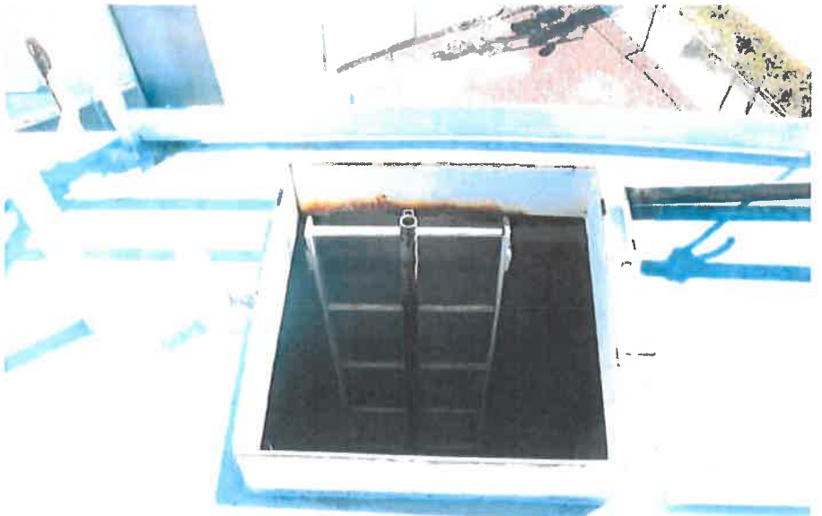
E-11 View of the roof hatch, illustrating corrosion along the top and bottom of the curb.
