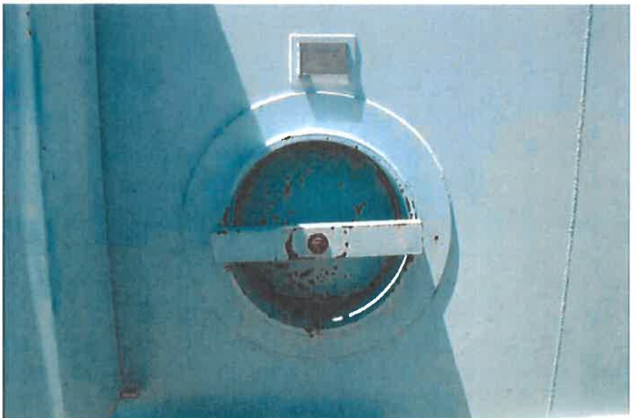
E-25 View of the manhole, illustrating corrosion on the cover and monobolt anchor.
