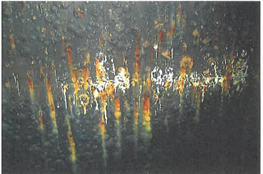
I-24 View of the shell, illustrating severe blistering, corrosion, and calcareous deposits present.
