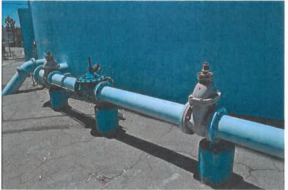
E-23 View of the inlet/outlet piping, illustrating mechanical damage and corrosion on the pipe flanges at the nuts and bolts.
