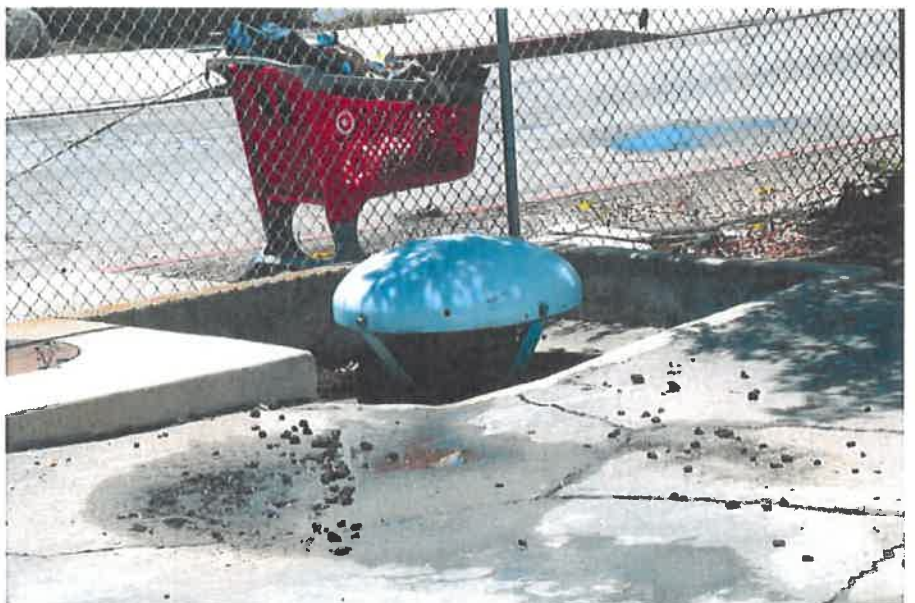
E-28 View of the overflow cover, illustrating delamination of the paint system on the cover.
