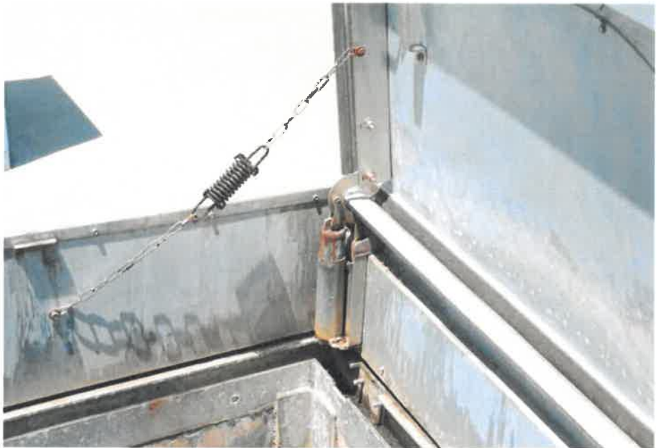
E-11 View of the roof hatch hardware, illustrating severe corrosion of the compression strut.
