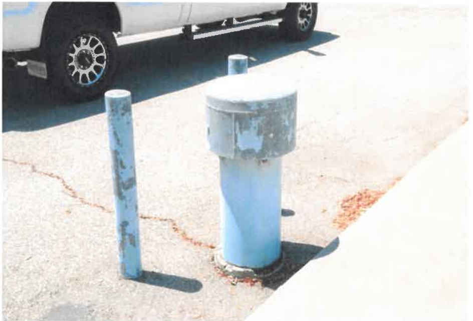
E-12 View of a vent pipe and bollards, illustrating delamination of the paint system on the vent pipe cover and bollards.
