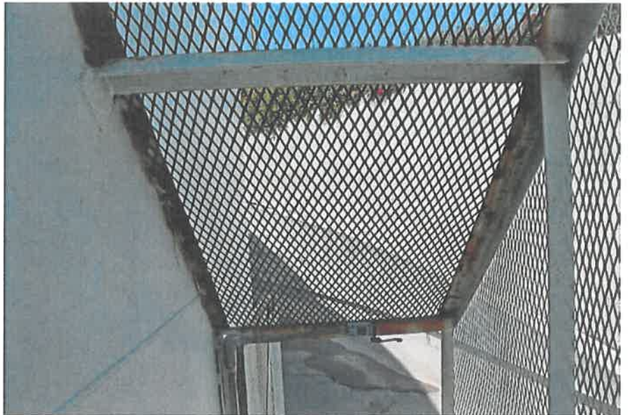
E-17 View of the underside of the vandal guard, illustrating corrosion along the perimeter angle.
