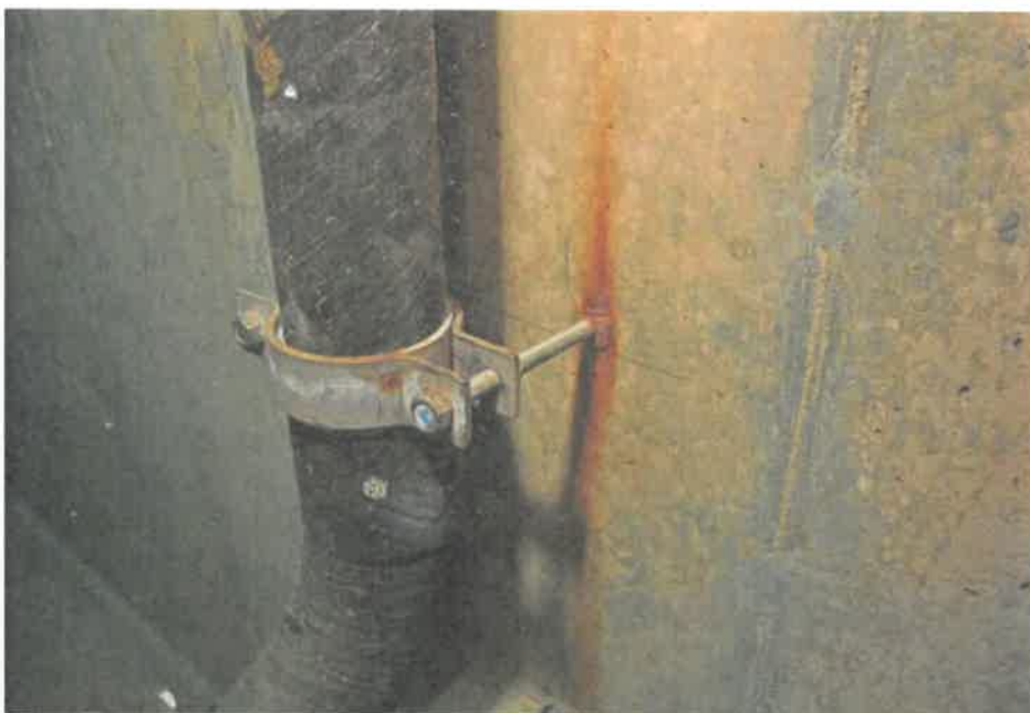
I-34 View of a pipe support, illustrating corrosion at the anchor bolt with staining present.
