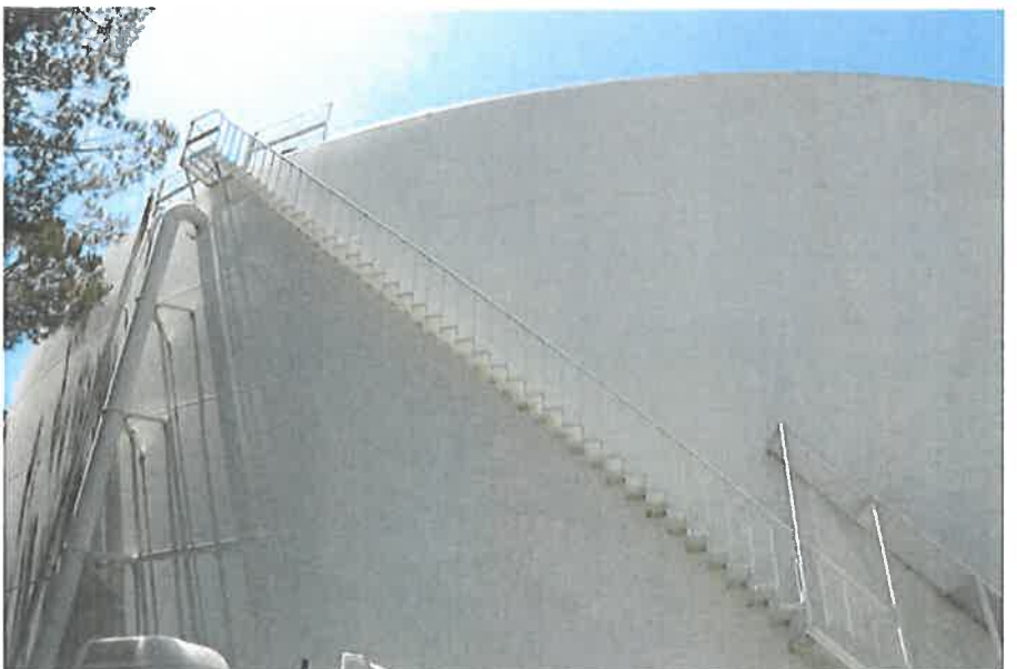
E-19 View of the stairway, illustrating severe oxidation and fading of the paint system on the stairway and adjacent shell.
