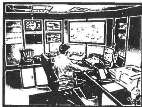
San Gabriel's Central Control Room
