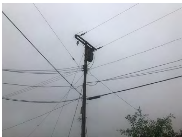
One (1) pole-mounted transformer
