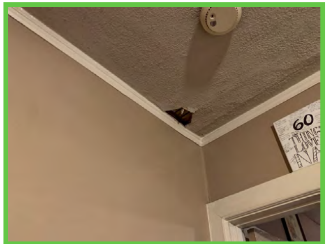
18) Ceiling finish and hole in ceiling
