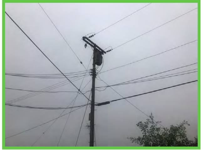
One (1) pole-mounted transformer 46
