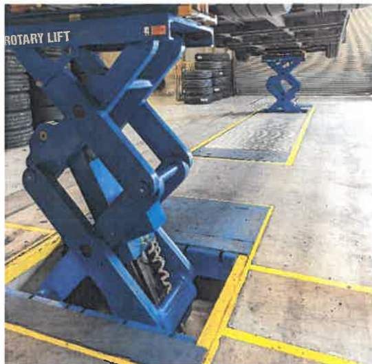
Figure 4: new bus hoists at Maintenance Bay 1
