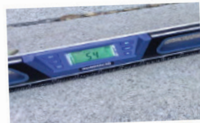
Excessive slope in perimeter concrete slabs.
