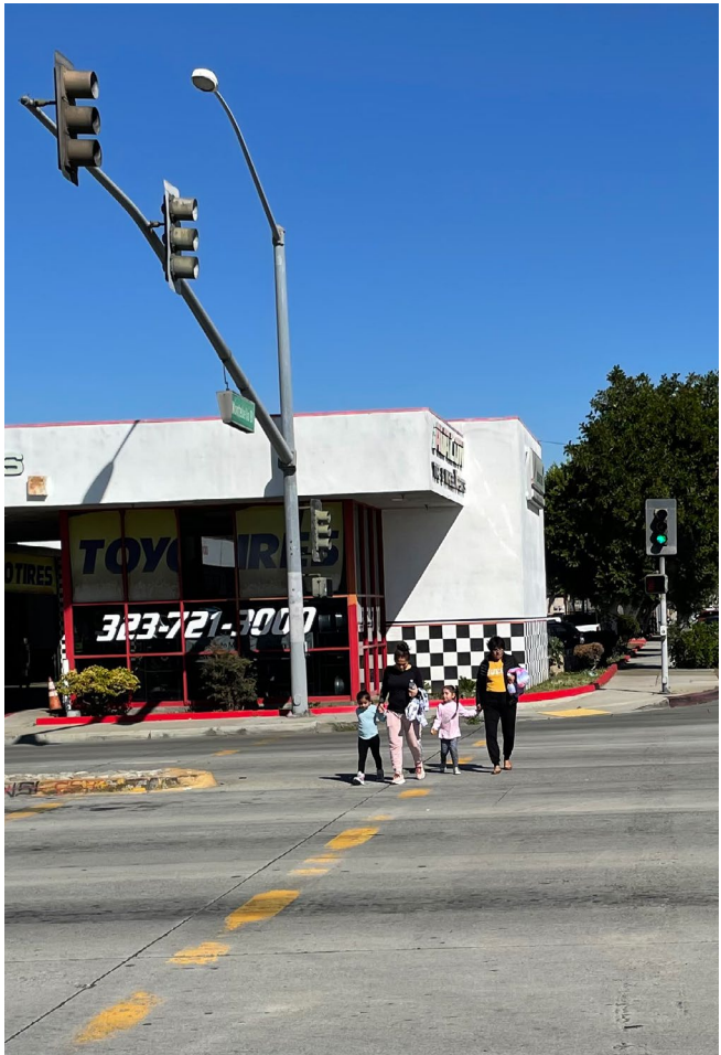
Faded Crosswalk markings at Montebello Boulevard and Washington Boulevard
