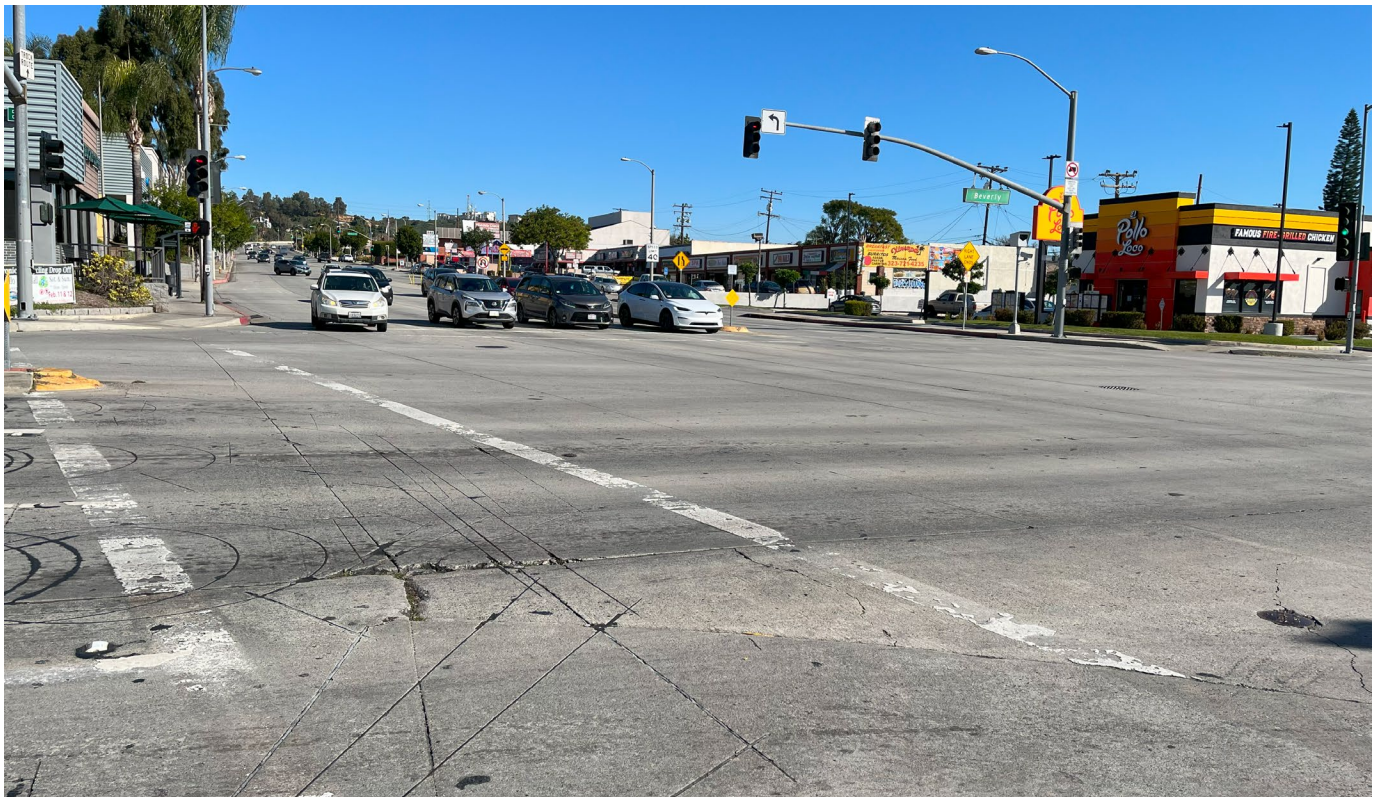
Faded crosswalk at Beverly Boulevard and Montebello Boulevard
