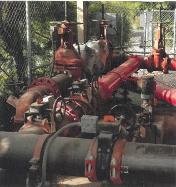
Outdated and Looming Infrastructure on Golf Course Needs Replacing
