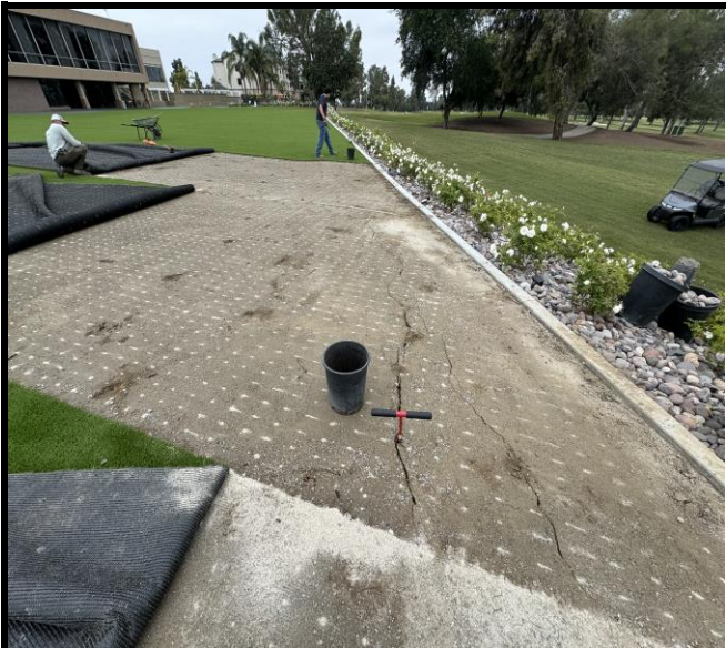
Cracks revealed in base layer. When probing soil beneath base we reached an average of 30 inches a probe
