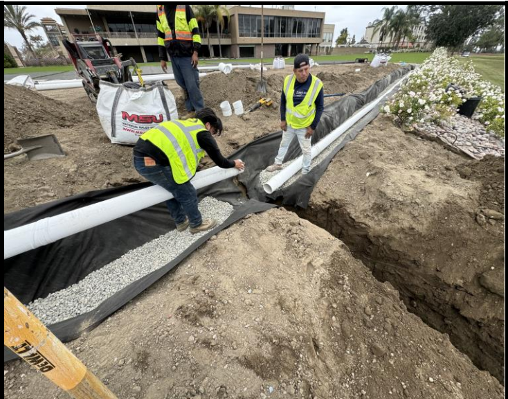
Pipes meeting at inlet
