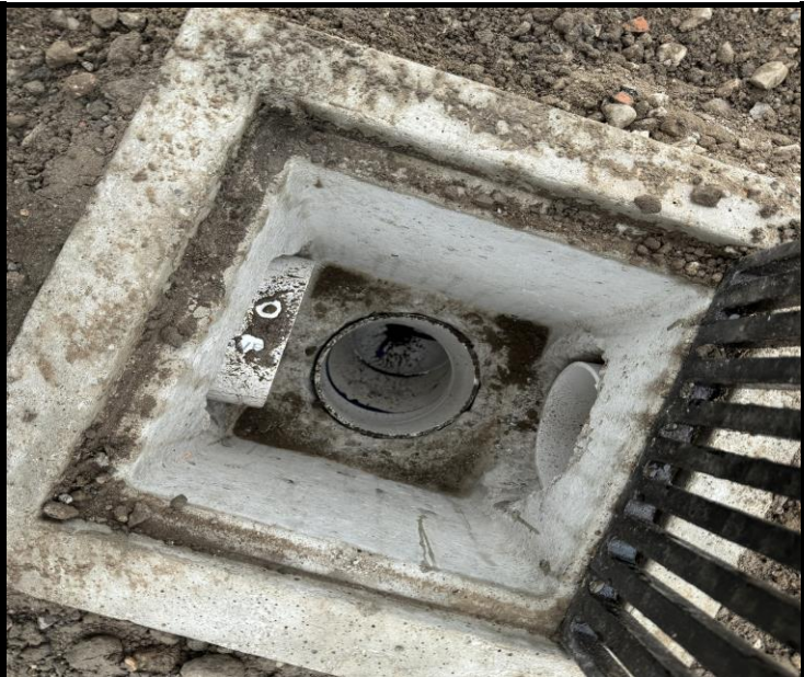
Drainage pipe rejected. 6 inch installed instead of 12 inch
