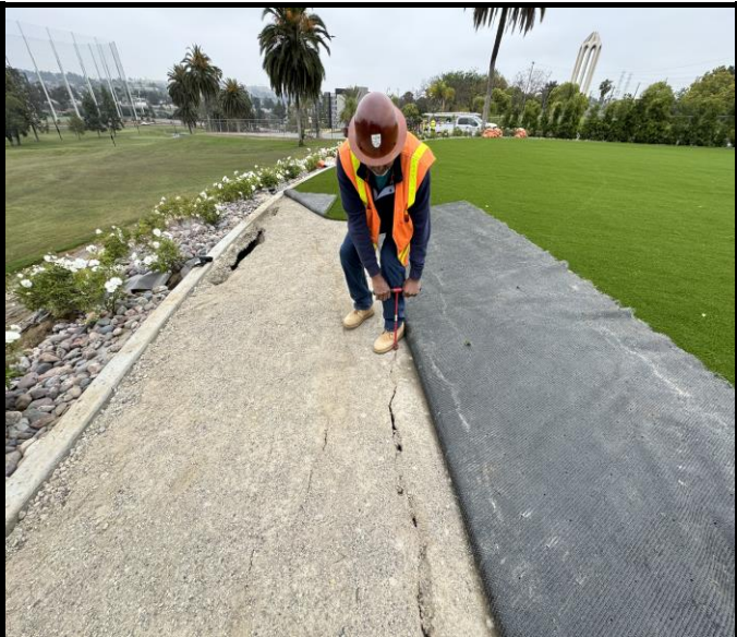
Cracks revealed in base layer. When probing soil beneath base we reached an average of 30 inches a probe
