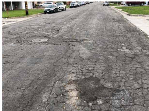
BEACH STREET: LOOKING EASTERLY (SHOWING PAVEMENT CONDITIONS)
